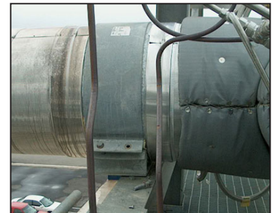
Previous Support Failure
